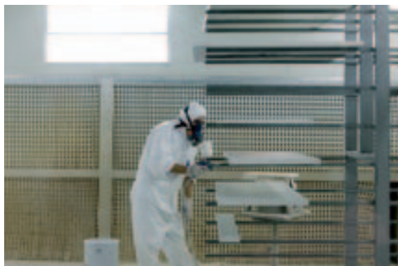
Spray painting should be conducted in a spray booth with an exhaust system that removes chemicals and effectively disperses vapours.
