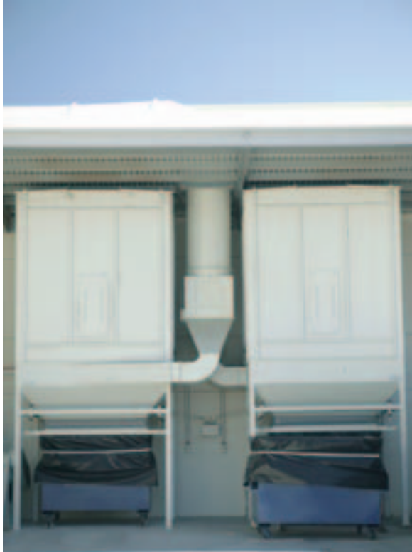
Centralised dust extraction system.
