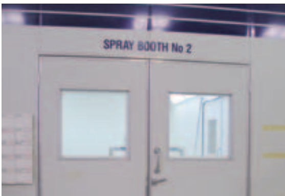
Are your spray booth doors securely closed during operation?
