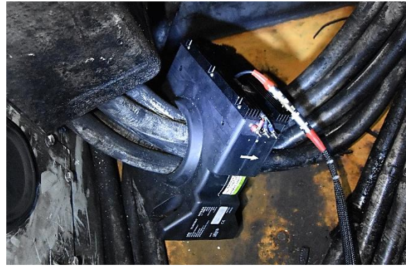
Current transducer on main DC generator
