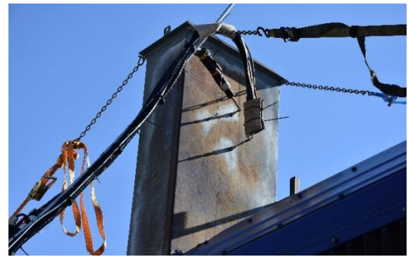
Exhaust stack and emissions sample probes on 8113
