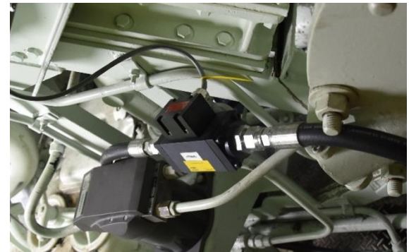
High precision fuel flow meter on return line
