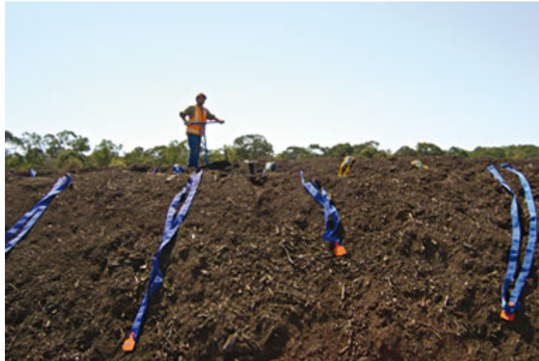
Figure 12. Illustration of the technique used to bury bags containing alligator weed in compost windrows at the experimental site.
