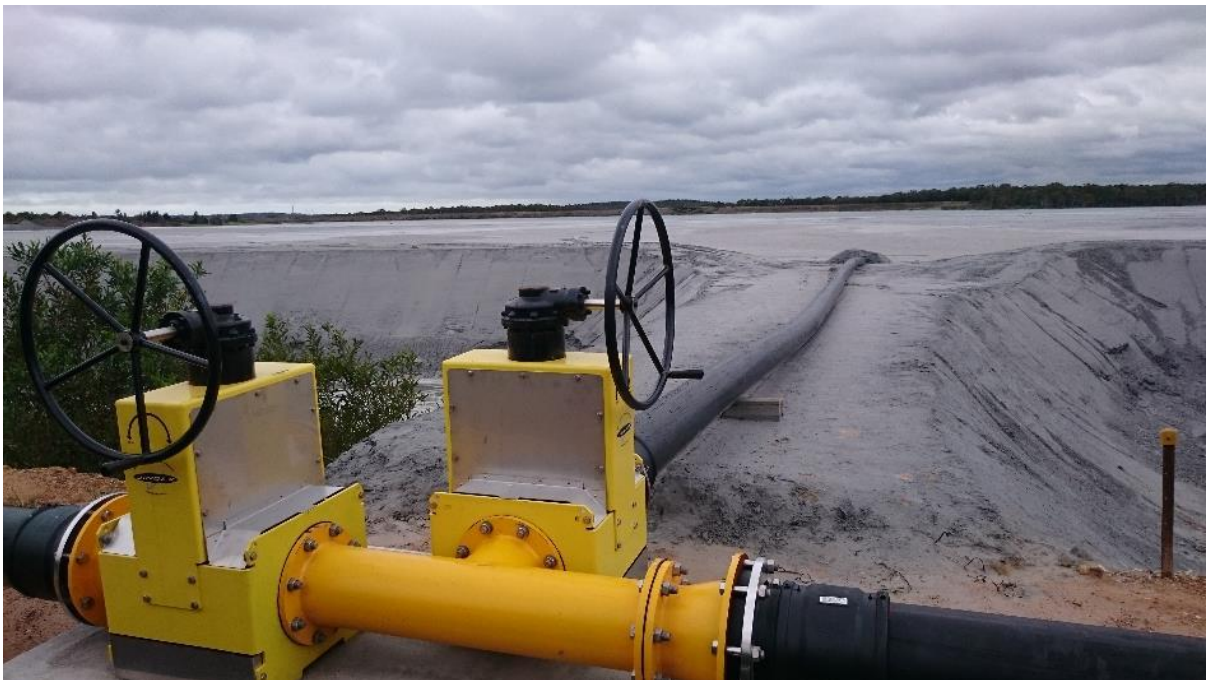
Figure 8: Ash slurry pipeline and valves to coal ash dam
