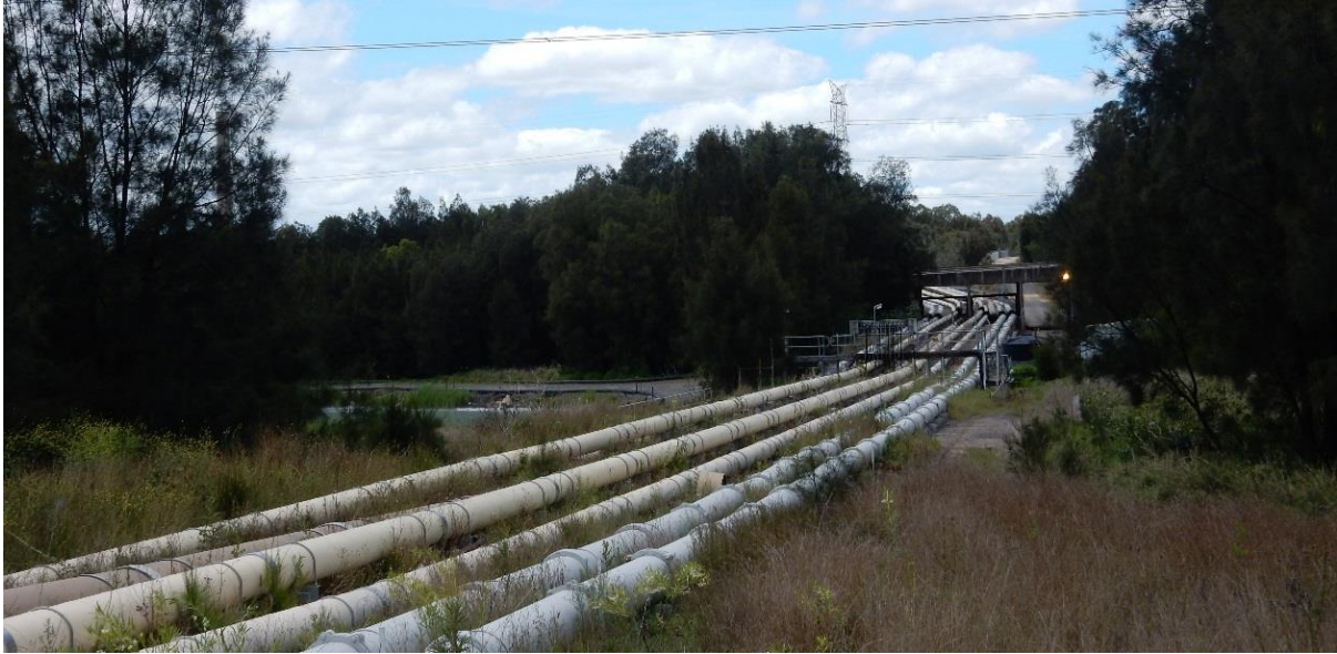
Figure 7: Pipelines for ash slurry
