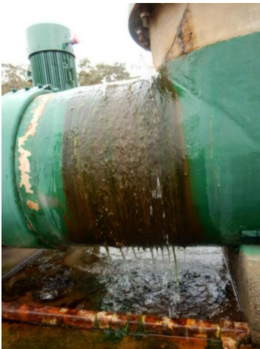
Figure 11: Return water pump manifold leak
