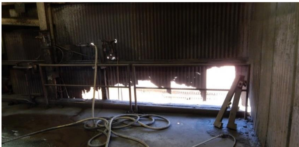
Photo 12: Degraded mill walls, allowing fugitive dust emissions
