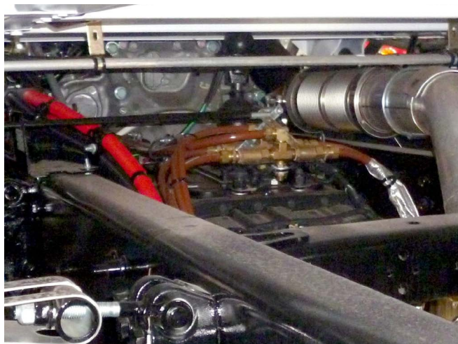
Fuel line (brown polyamide tubes) positioned close to the exhaust pipe. Further shielding may be required. Photo: Peter Hart/Hartwood Consulting
