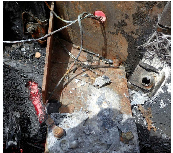
Hot terminals can occur on minor or major circuits. In this case the return connection in a beacon light was poor because the rubber mount was not tight. Photo: Peter Hart/Hartwood Consulting
