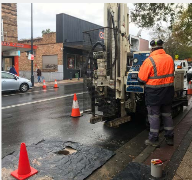
Preparing the drill rig and location for groundwater monitoring well installation at Jannali. Photo: EPA
