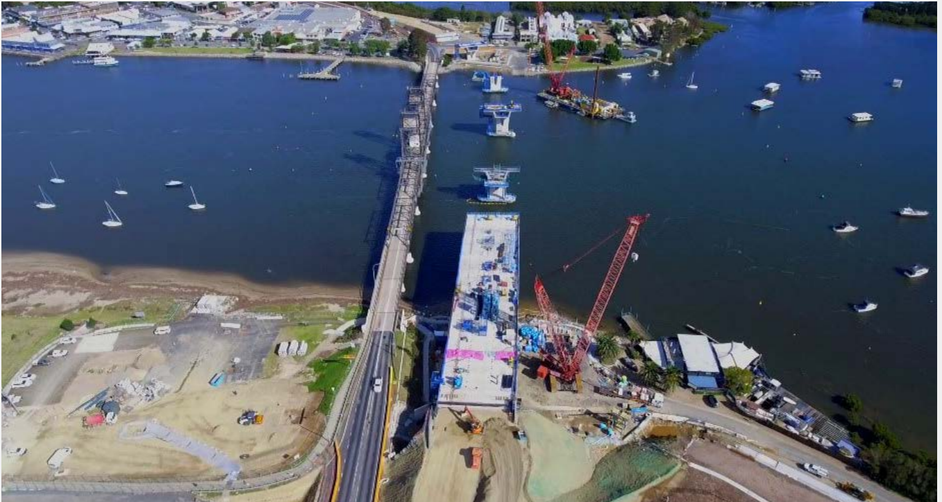
First spans being installed for the new Batemans Bay Bridge over Clyde River. Photo: Transport for NSW
