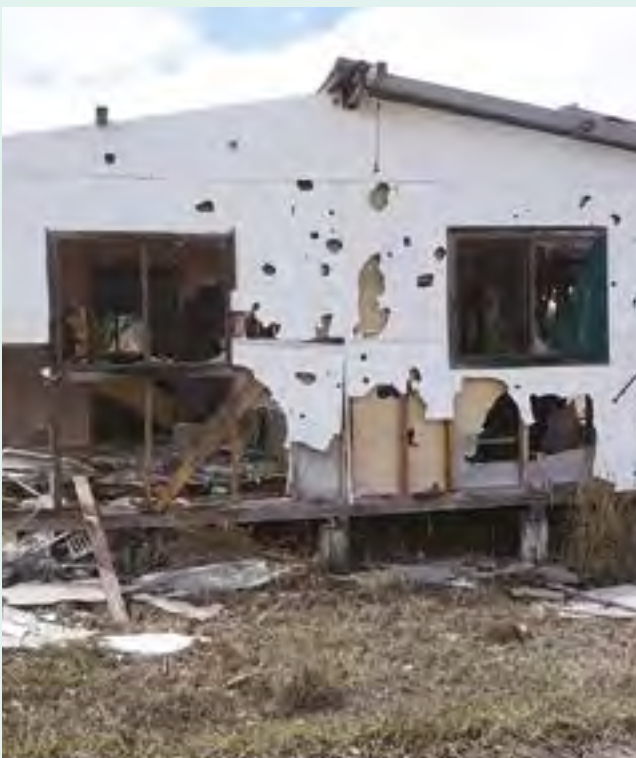
Abandoned asbestos house on Baryulgil Community, NSW Photo: Keith Bolton
