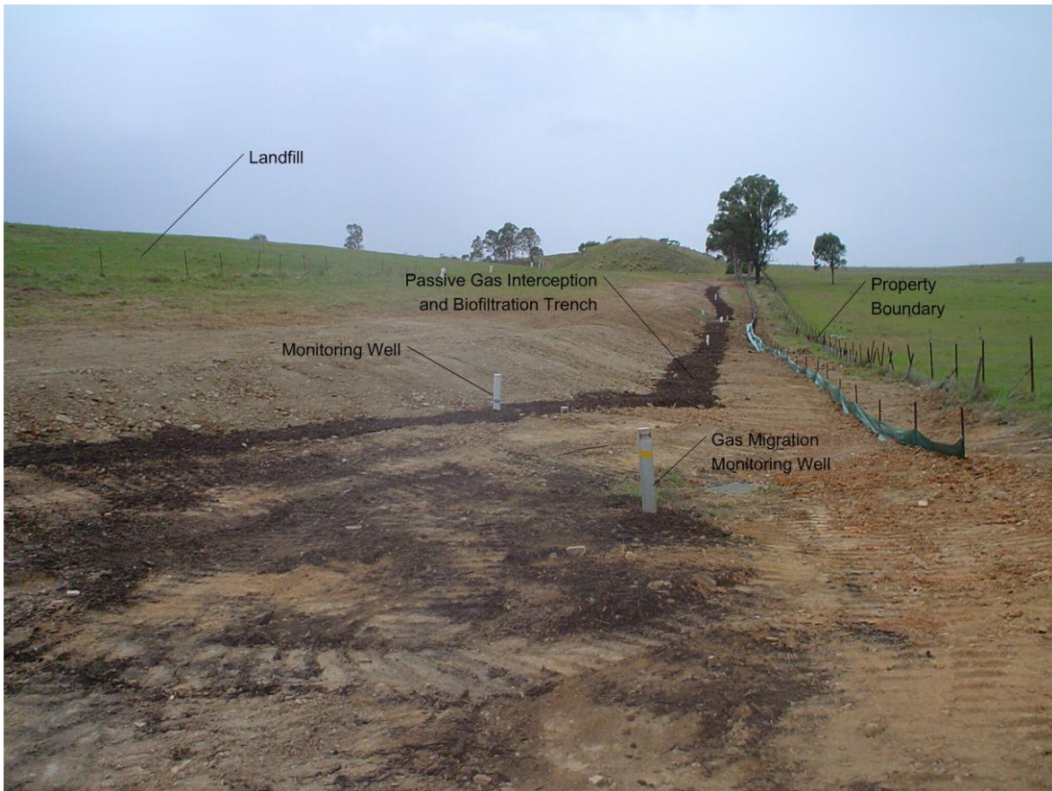
Figure 21: Photograph of passive gas interception and biofiltration trench
