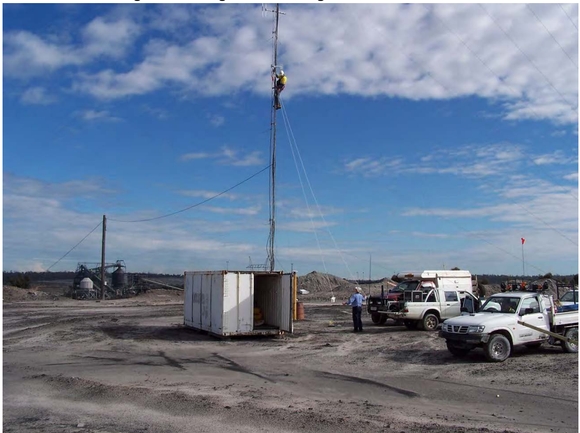
Figure 1 - Ewington Meteorological Station
