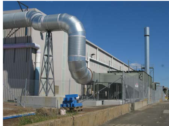
Temporary emission control enclosure, former Orica chlor-alkali plant. Photo: M Hart, EPA
