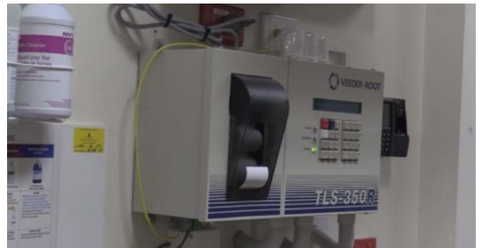
Automatic tank gauge (ATG)
