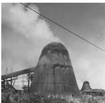
Old tepee in poor condition
