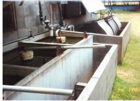
Piggery flushing tanks
